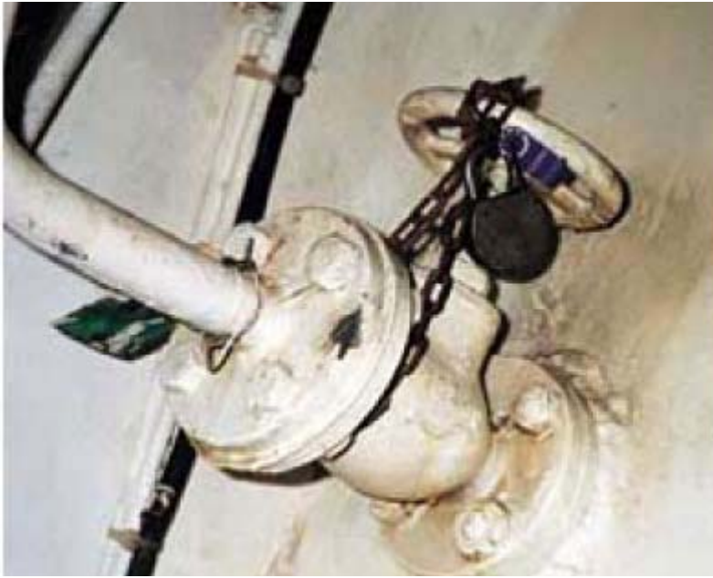
Locking of overboard discharge valve in port.
